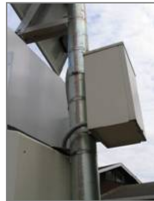
Pole-mounted battery box
